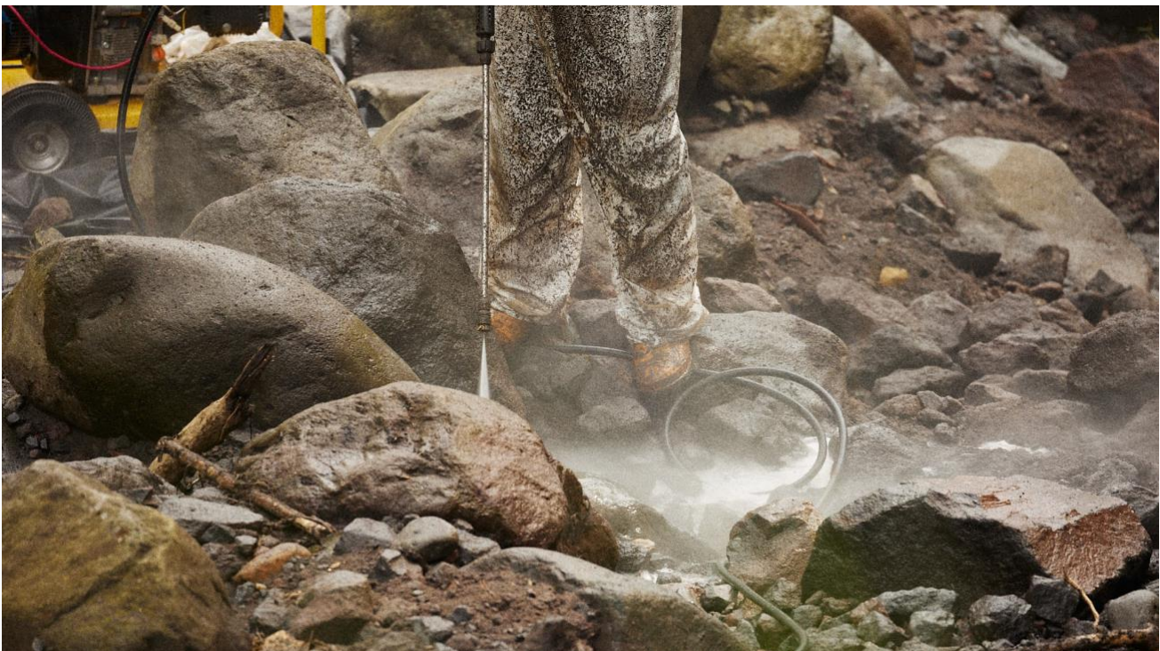
OCP Pipeline Rupture, January 2022. © Mauricio Rosenfeld/Amazon Watch
